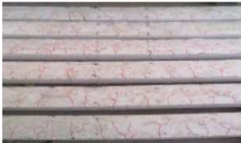
Fig 7. Crack pattern at middle of the beams
